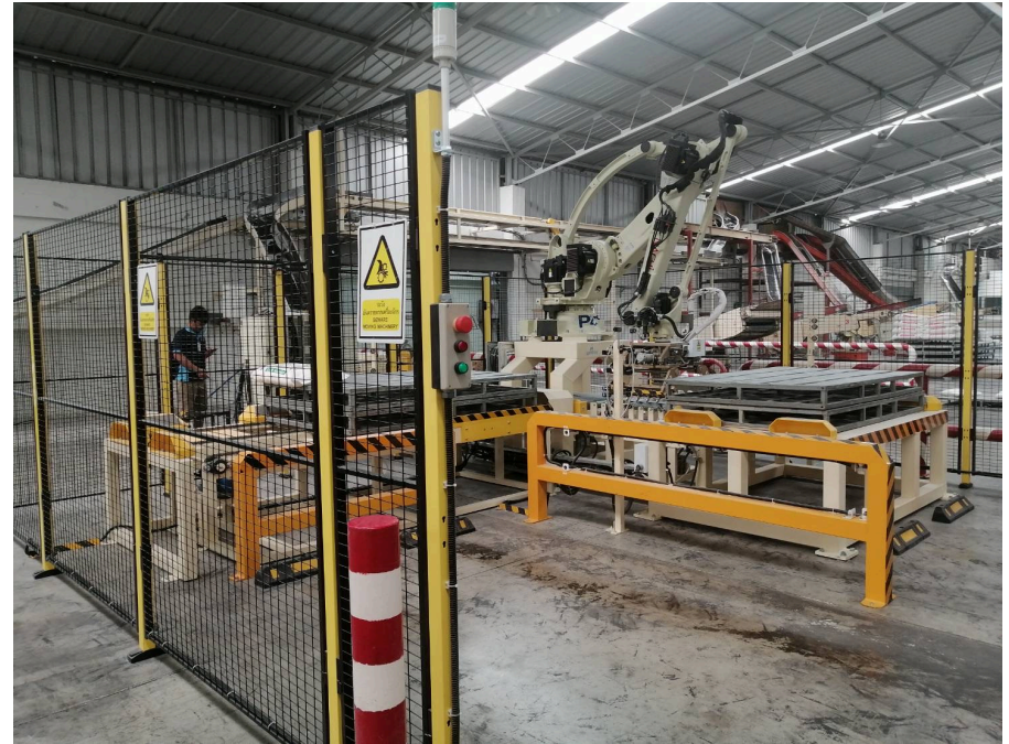
COMPANY : UNITED FLOUR MILL ( Line P3 )
