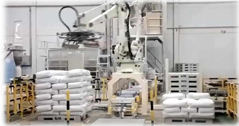
COMPANY : SINOE STARCH Line No.2
