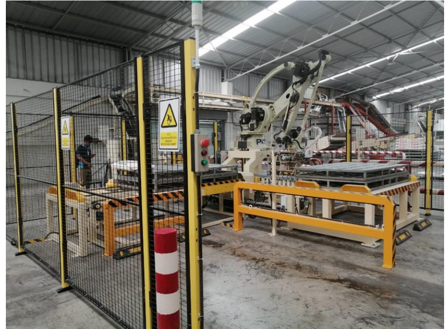
COMPANY : UNITED FLOUR MILL ( Line P3 )
